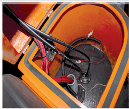
PIPE FOR ENGINE WIRES (INSIDE OF CONSOLE)
