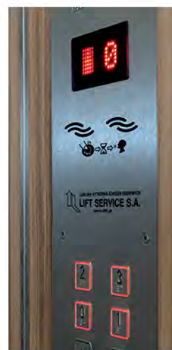
CONTROL OPERATING CASSETTE
