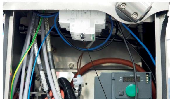
Earth leakage circuit breaker test button
